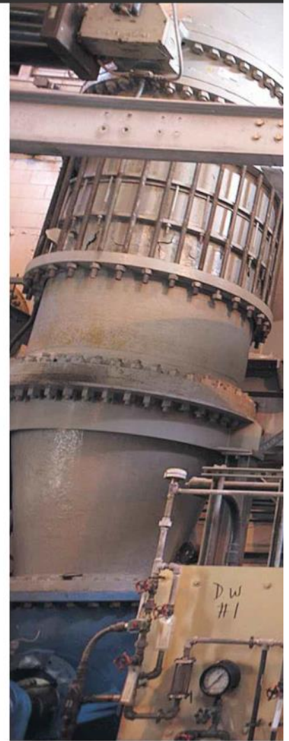
Electrical equipment powering these huge pumps at the Bay Park sewage treatment plant was damaged by a tidal surge during superstorm Sandy.
